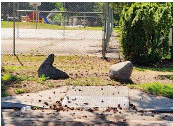
Figure 20. Underhill Park curb ramp without accessible route to facilities.
