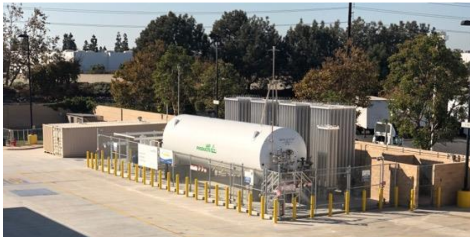
Figure 32: Hydrogen Storage and Dispensing Examples
