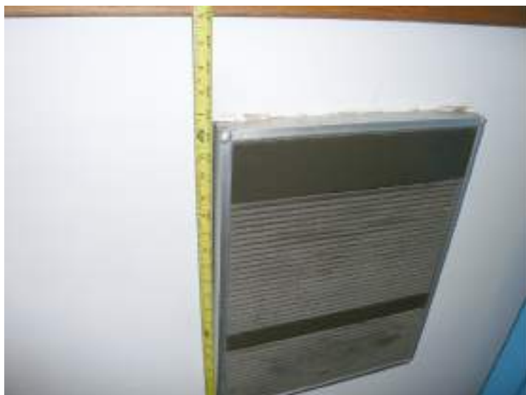
ELECTRICAL HEATER TO BE REMOVED. CONTRACTOR TO INFILL HOLE WITH NEW GYPSUM BOARD, PATCH AND PAINT WALL ENTIRELY TO MATCH EXISTING WALL
